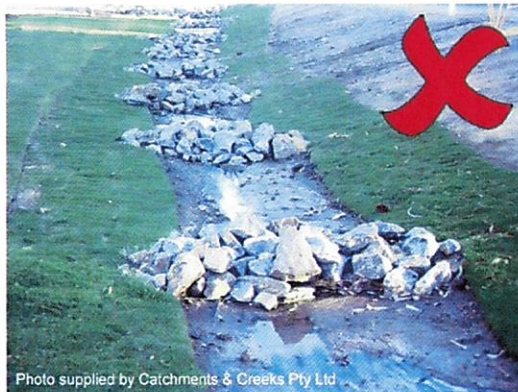
Photo 7 – Poor placement of rocks, note rocks are higher in centre of check dam
