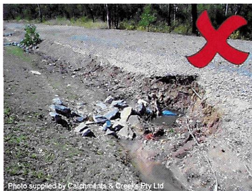
Photo 9 – Typical erosion problem when placed in dispersive soil
