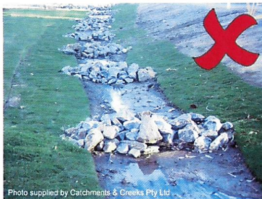
Photo 7 – Poor placement of rocks, note rocks are higher in centre of check dam
