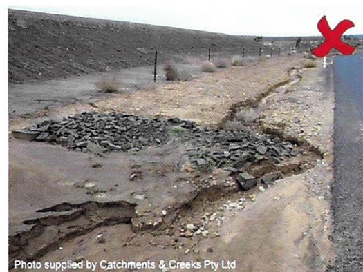
Photo 10 – Typical erosion problem when placed in dispersive soil
