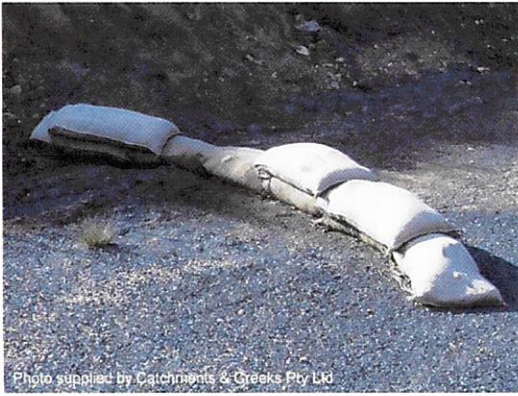
Photo 3 – Sandbag check dam
